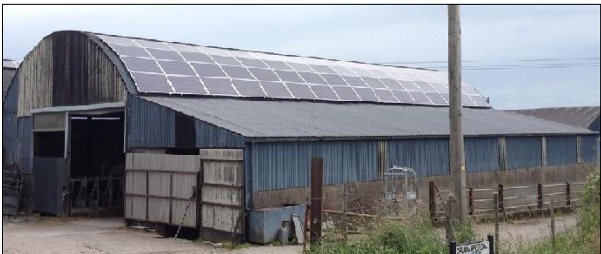
Fig.1 PV array fixed to the roof of the cattle shed
